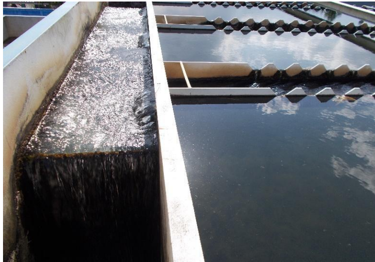
Gambar 3.12 Unit Filter PDAM Intan Banjar
