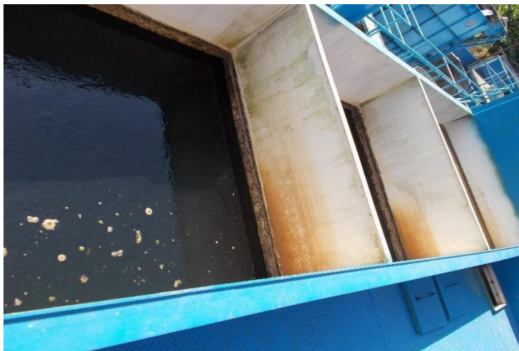
Gambar 3.13 Unit Sedimentasi PDAM Intan Banjar
