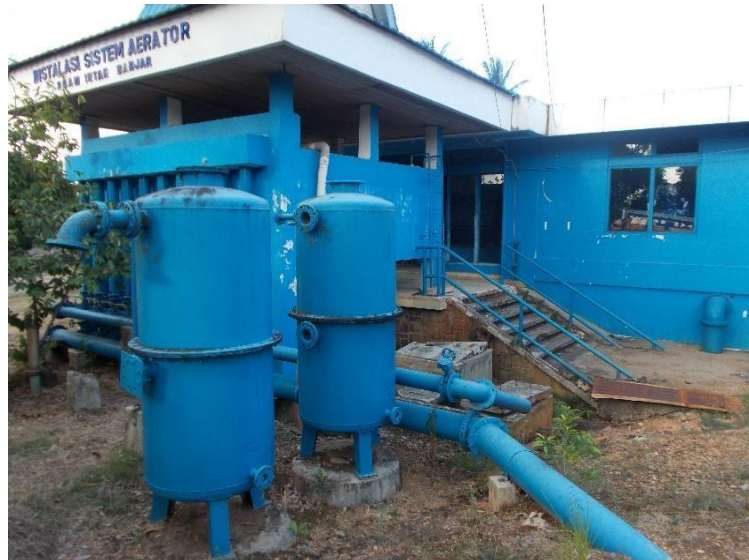
Gambar 3.28 Pipa Distribusi (transmisi) IPA I STM (Aerator)
