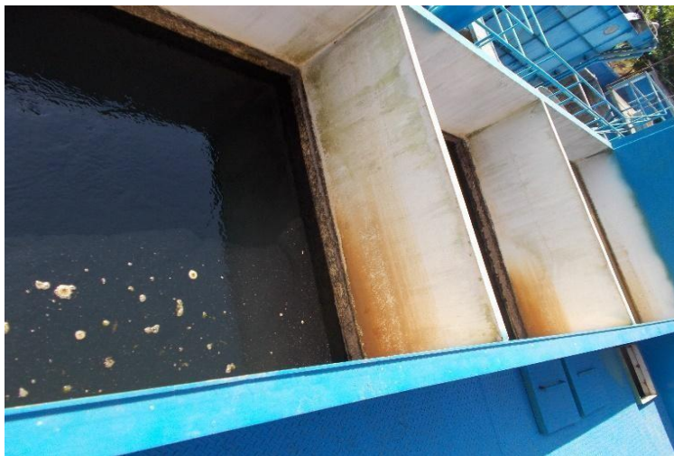
Gambar 3.13 Unit Sedimentasi PDAM Intan Banjar
